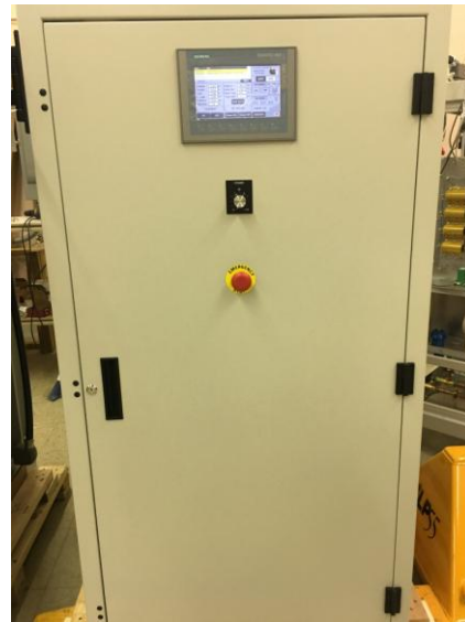
Fig.5. General view of the APT-100-3 DC module with advanced control system
